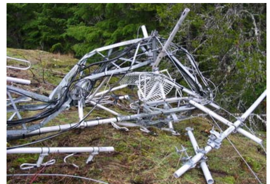
The toppled tower and former antennas transformed into a pile of scrap metal
