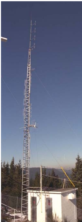
WARA Main Repeater Tower during better times!
